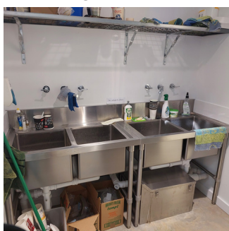
Left: the large sinks purchased with fit-out funding have already been well utilised.
